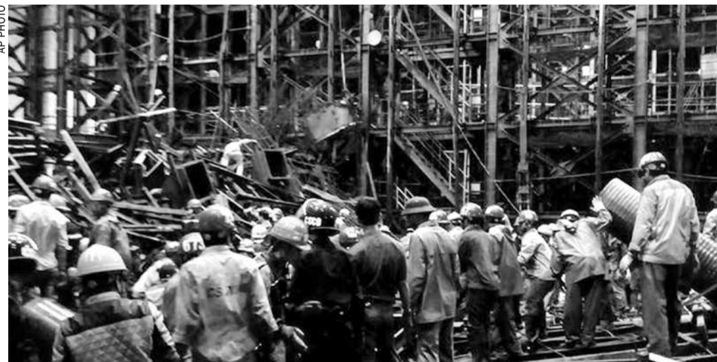
Rescuers work through the rubble trying to find survivors after scaffolding collapsed in an economic zone in Ha Tinh province in central Vietnam
