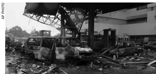
The remaining structure of a gas station after it exploded in Accra
