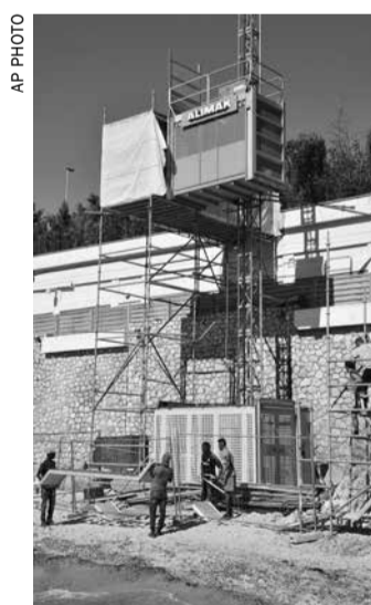
Workers dismantle a temporary elevator on the public beach called "La Mirandole" located below a mansion owned by the Saudi royal family in Golfe Juan Vallauris, southeastern France
