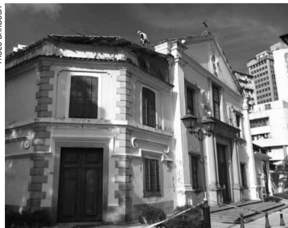
A section of the roof of Saint Augustine Church collapsed on Sunday while a mass service was being held. No one is reported to be injured, since the room the roof fell in was not being used at the time. The site was inspected yesterday by the Cultural Affairs Bureau president, Ung Vai Meng, and workers have started to repair the roof. The area facing the church, which is one of UNESCO's world heritage sites in Macau, has been sealed.
