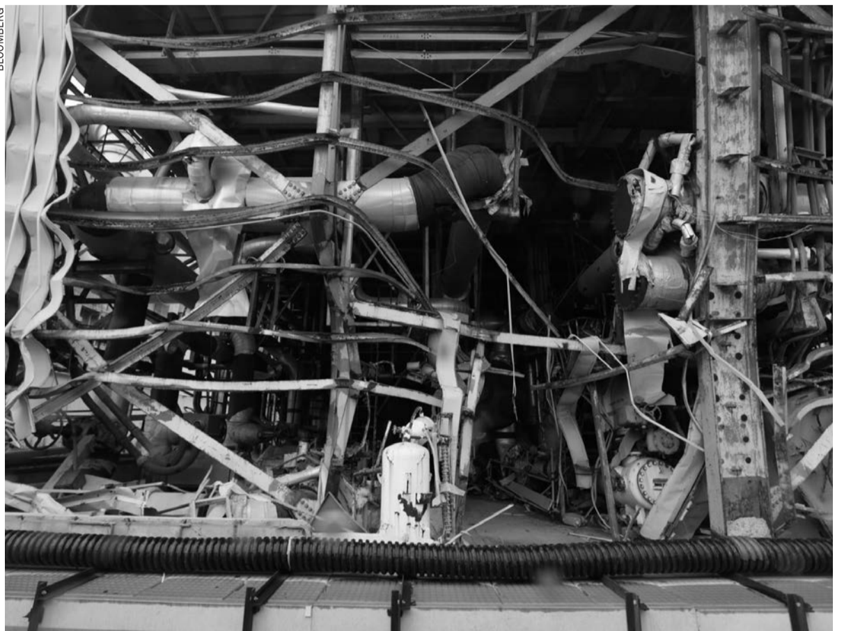
The damaged building housing the No. 4 reactor is seen from coastal side at Tokyo Electric Power Co.'s (Tepco) Fukushima Dai-ichi nuclear power plant
