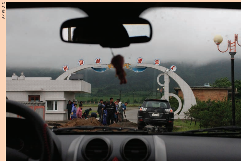
Workers fix the access road to Pipa Island, a tourist attraction inside the Rason Special Economic Zone
