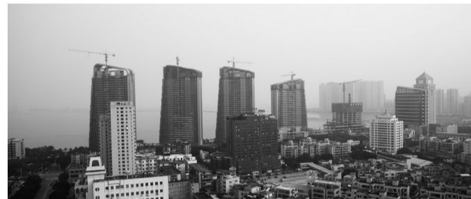
Cranes operate at a residential construction site in the Gongbei district of Zhuhai
