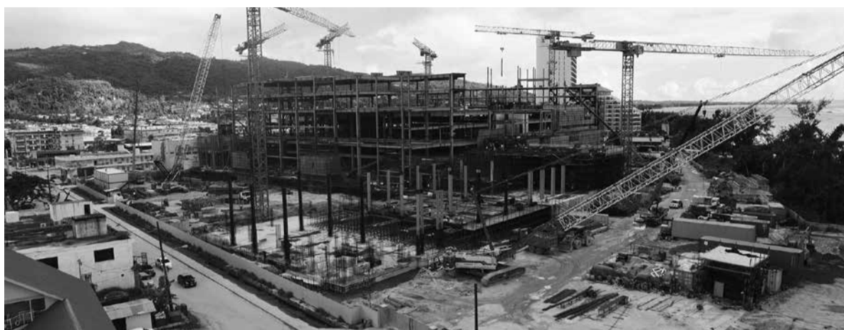
Cranes and equipment stand on the construction site of an integrated resort owned by Imperial Pacific in Saipan, September 2016
