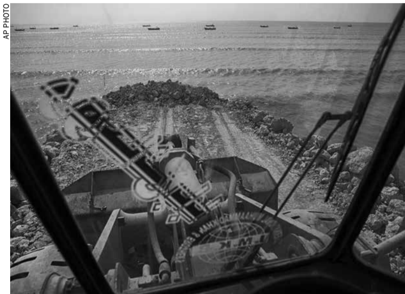
A bulldozer operates on a development site at Marine Drive in Gwadar, Pakistan
