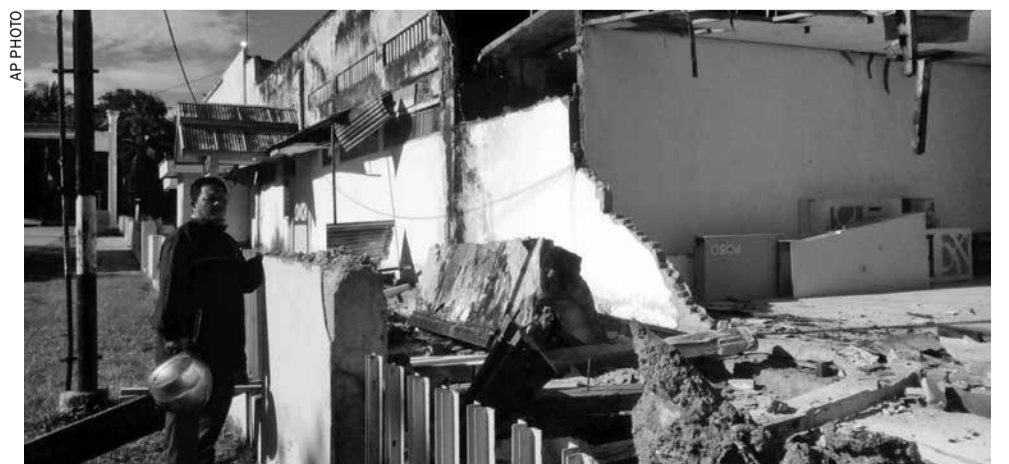
Damage caused by an earthquake in Poso, Central Sulawesi, Indonesia, on May 30
