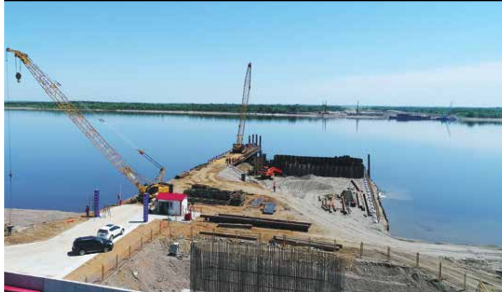
The construction site of Heihe-Blagoveshchensk road bridge at the border of China and Russia. A 19.9km highway bridge connecting China and Russia over the Heilongjiang River is under construction. The road bridge is scheduled to open to traffic in October 2019.
