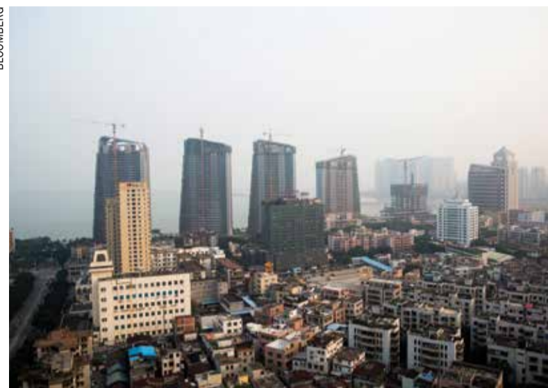
Cranes operate at a residential construction site in the Gongbei district of Zhuhai
