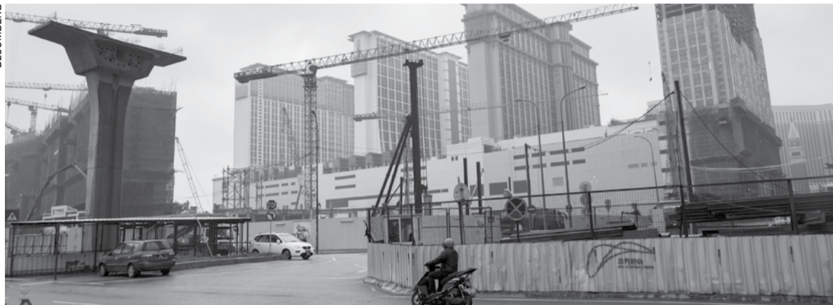
A pylon for an elevated track for the LRT stands under construction near Sands China Ltd.'s Sands Cotai Central casino resort
