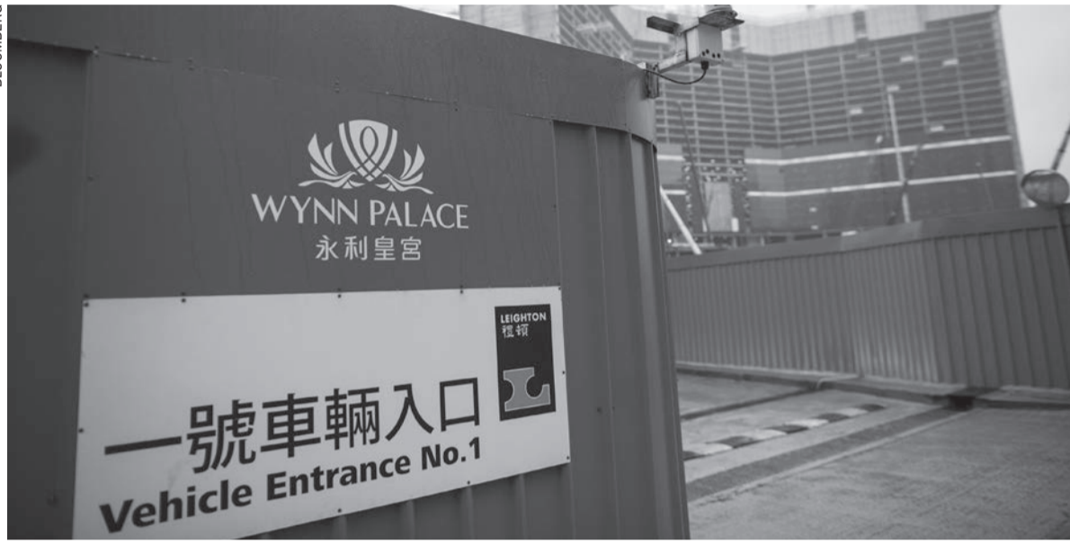
Signage for the Wynn Palace project, developed by Wynn Resorts Ltd., is displayed at an entry gate to the construction site
