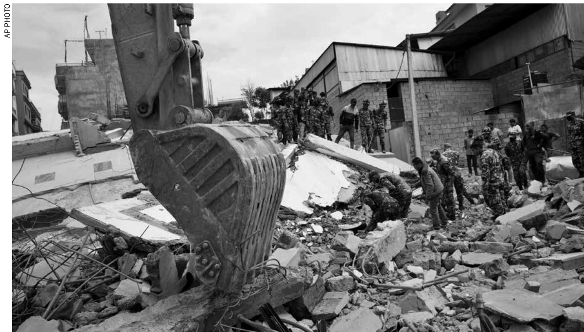
Nepalese security personnel engage themselves in a rescue operation at the site of a budget hotel that collapsed in Saturday's earthquake, in the Kalanki neighborhood of Kathmandu
