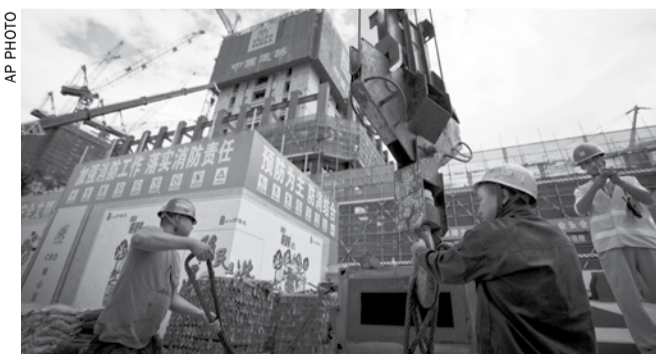
Workers load a steel frame outside a construction site at the Central Business District of Beijing
