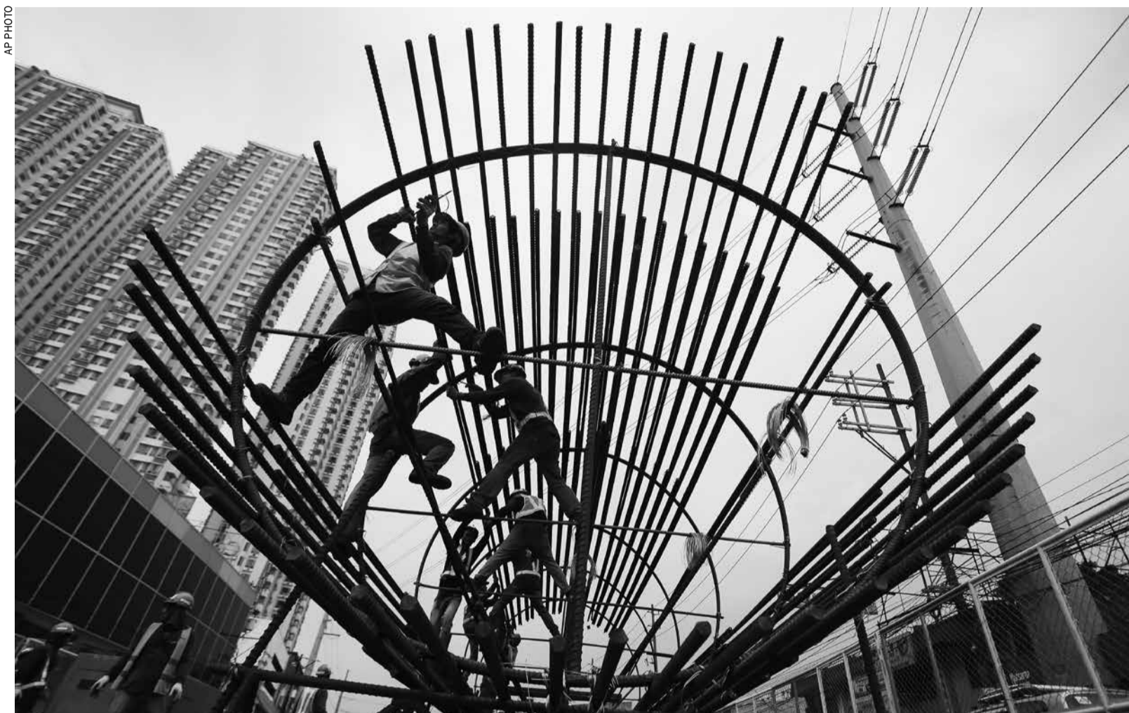
Filipino workers arrange metal rods at a government road project in suburban Quezon City, north of Manila, Philippines
