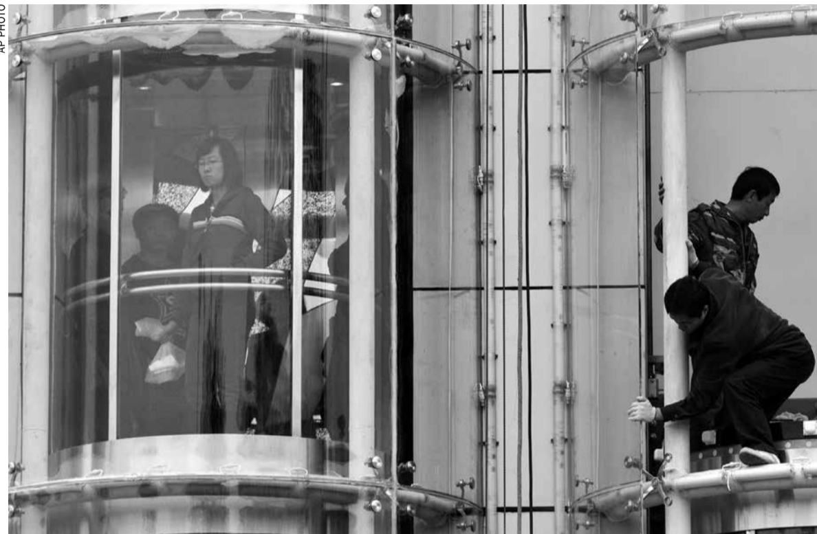
Workers, right, prepare to install a piece of glass wall covering an elevator tunnel while a woman, left, looks down from a descending elevator in Beijing
