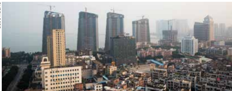
Cranes operate at a residential construction site in the Gongbei district of Zhuhai
