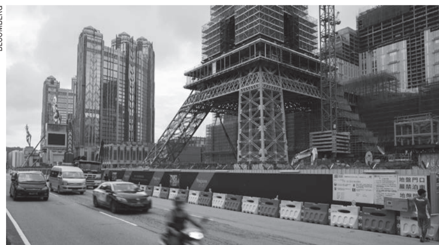
Traffic drives past a half-sized replica of the Eiffel Tower stands at the construction site of Parisian Macao, operated by Sands China
