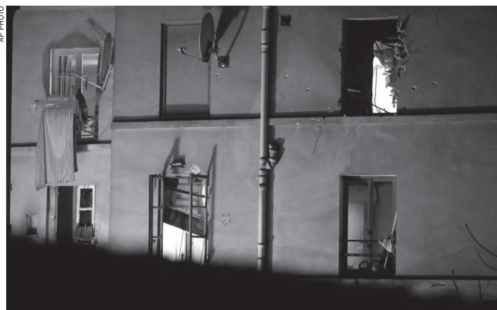
Bullet holes and smashed windows are pictured on the back side of the house after an intervention of security forces against a group of extremists in Saint-Denis, near Paris
