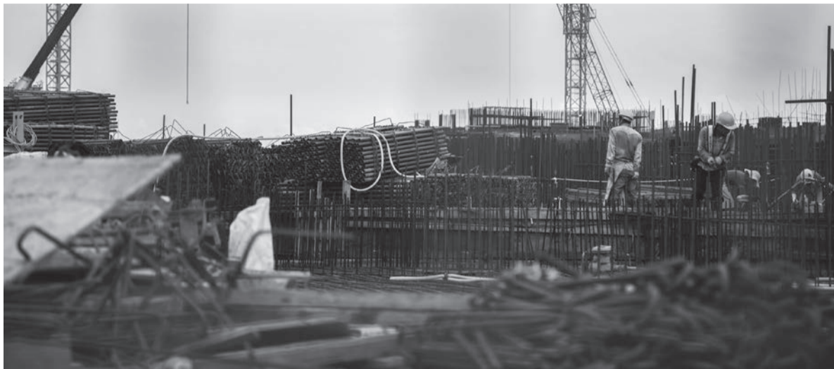
Workers labor as cranes operate at the Lisboa Palace construction site, developed by SJM in Macau
