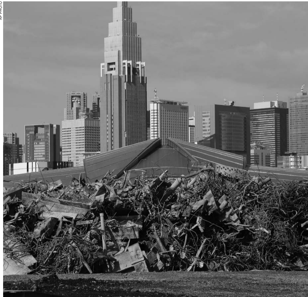
Skyscrapers are seen above the roof of the Tokyo Metropolitan Gymnasium as the rubble of Japan's National Stadium, demolished to build a new Olympic Stadium, is collected at one corner of the vacant site
