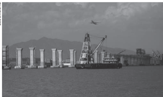
A transport barge travels past the under construction Delta Bridge as an aircraft takes off from HK airport
