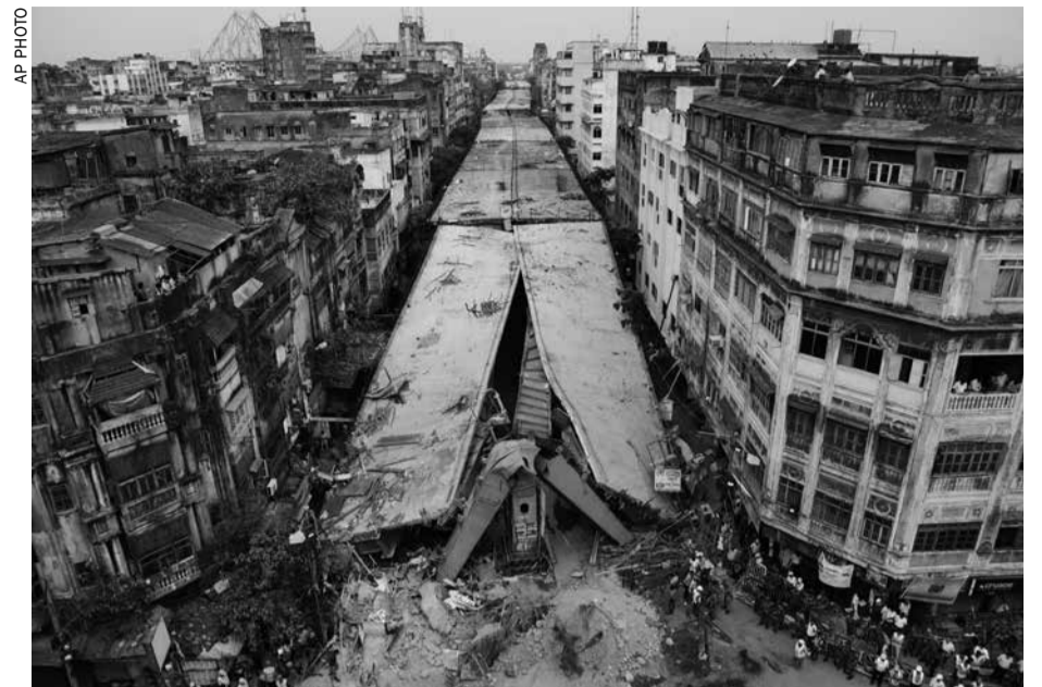
General view shows a partially collapsed overpass in Kolkata, India
