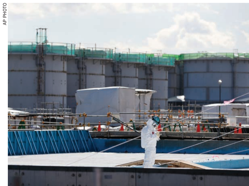
A worker, wearing protective suits and masks, takes notes in front of storage tanks for radioactive water at the tsunami-crippled Fukushima Dai-ichi nuclear power plant, operated by Tokyo Electric Power Co. (TEPCO), in Okuma
