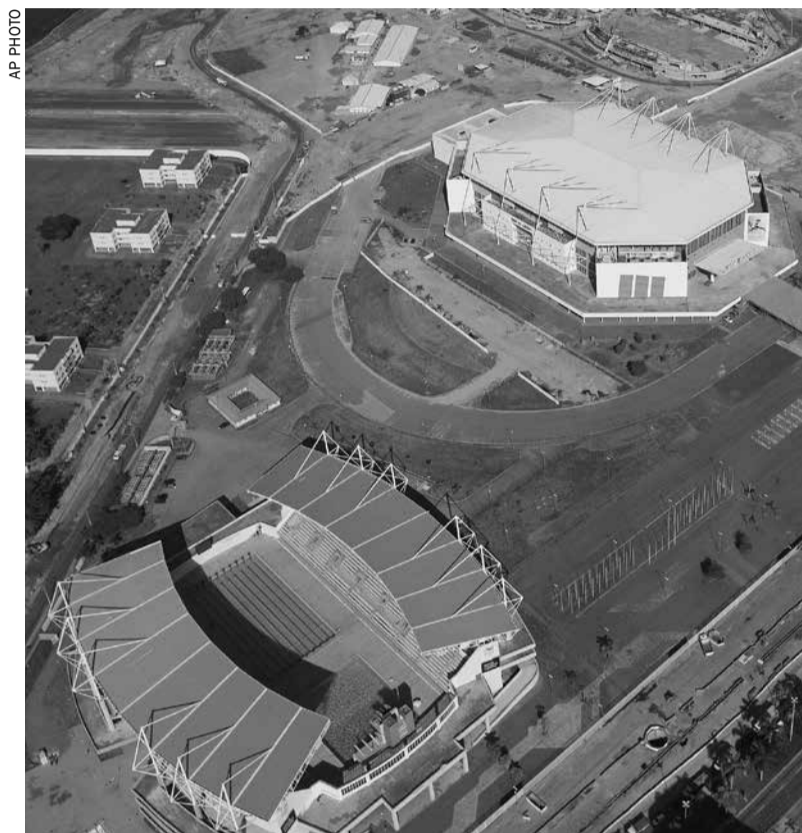
This June 27, 2014 file photo, shows the Olympic Arena (top) and the Maria Lenk Aquatics Center under construction in Rio de Janeiro
