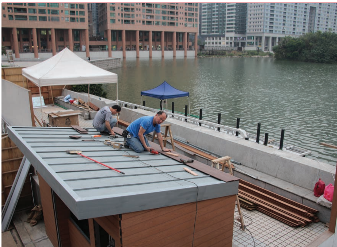
Construction in progress near Nam Van Lake. During the December 2015 Policy Address presentation, the Secretary for Social Affairs and Culture, Alexis Tam, announced that the area abutting the lake – which is near the government headquarters – will have cafes with outdoor zones managed by the Cultural Affairs Bureau.
