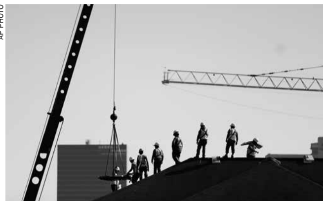
Construction workers unload supplies off a hoisted pallet on a rooftop in Atlanta
