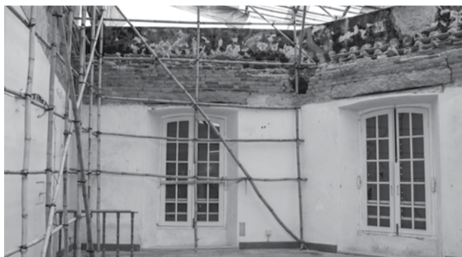
Damaged structures at Saint Augustine Church
