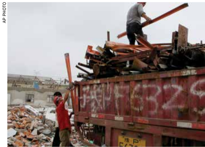
Scrap collectors load materials into a truck on the site of demolished factories in Zhoupu Township in Pudong district of Shanghai
