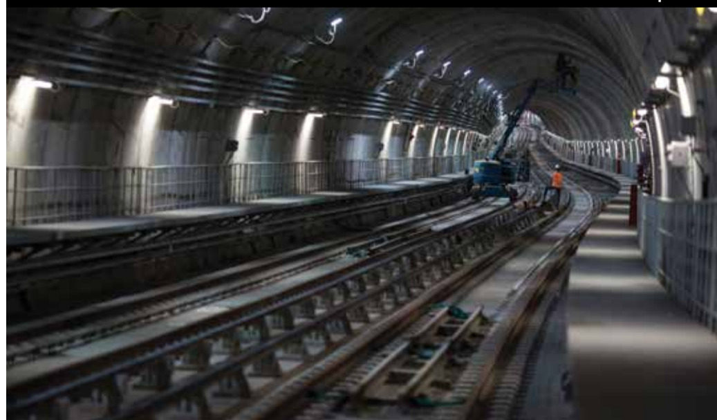
Men work in the new underground subway tunnel below Ipanema neighborhood in Rio de Janeiro, Brazil. Last-minute construction on the line has created fears after an April bike lane collapse that plunged two joggers to their deaths. An ocean-front section of the lane, an Olympic beautification project inaugurated in January, collapsed into a heap of broken cement when struck by a large wave.
