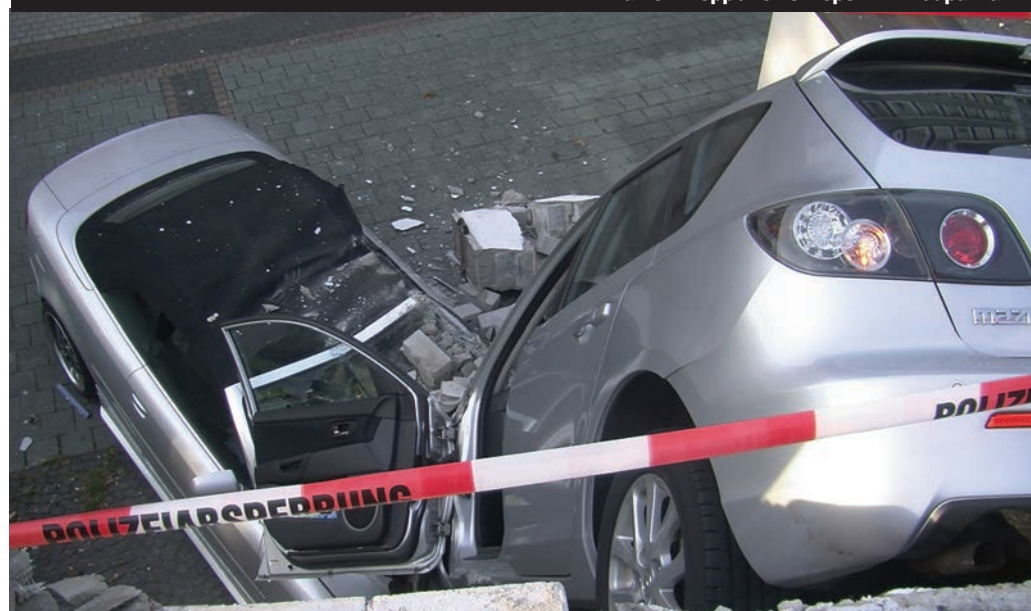
Car cash. An 80-year-old woman took an unintended short cut as she tried to drive her car (right) out of a multistory car park in Germany, breaking through the building's wall and landing on a parked convertible 3 meters below. Neither the driver nor her husband, 85, who was standing next to the car at the time, were hurt in the accident in Bottrop, Germany yesterday [Macau time]. The accident caused USD27,900 in damage.
