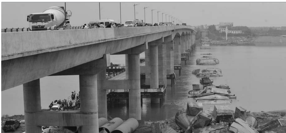
A bridge in the eastern province of Jiangxi collapsed yesterday while it was being dismantled, injuring five and leaving three missing. The collapse happened at around 9 a.m. in Taihe County. Three of the eight workers who fell into the river remain unaccounted for, according to the local government. The five who sustained injuries have been admitted to hospital.
