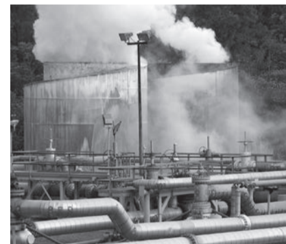
Chevron Corp.'s geothermal power plant operates in Salak, Indonesia
