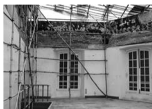
Back in May, the roof of the Saint Augustine Church partially collapsed
