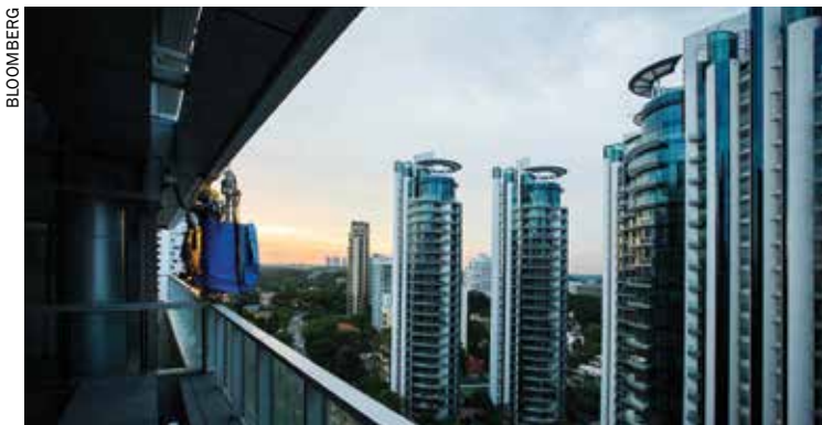
A worker rides a suspended platform as he performs construction work at a residential building in Singapore
