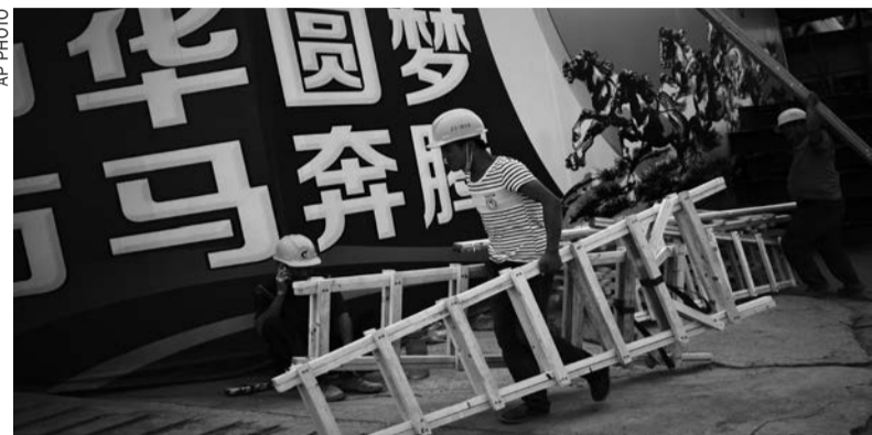
Workers carry wooden latter past by a Chinese government's propaganda "China Dream" billboard on display outside a construction side in Beijing
