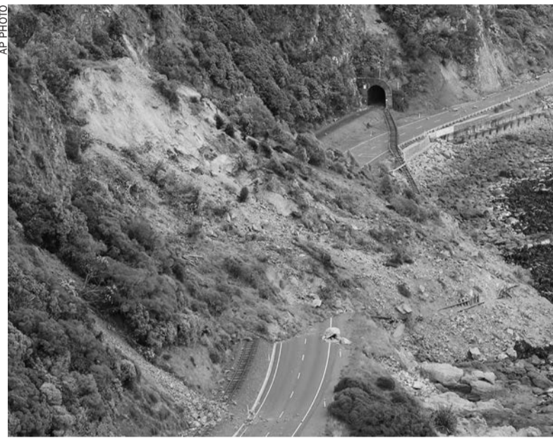
A landslide blocks State Highway One and the main trunk railway line north of Kaikoura
