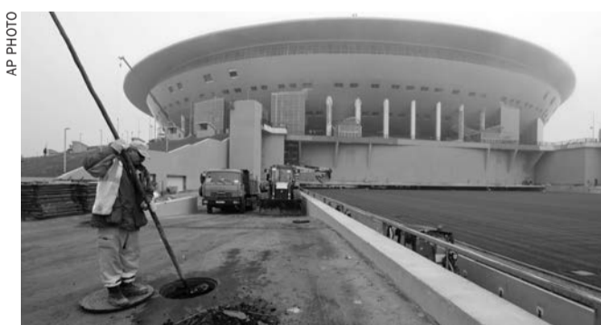
A worker cleans sewers near the retractable football pitch at the soccer stadium, which is under construction on Krestovsky Island, in St. Petersburg
