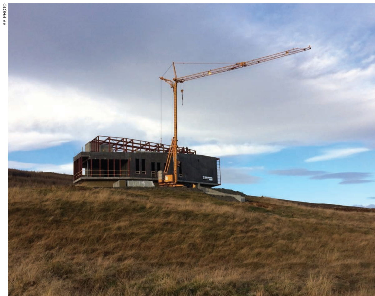
China's Arctic ambitions take shape at the construction site of the Aurora Observatory, a research facility to study the Northern Lights, in Karholl, Iceland
