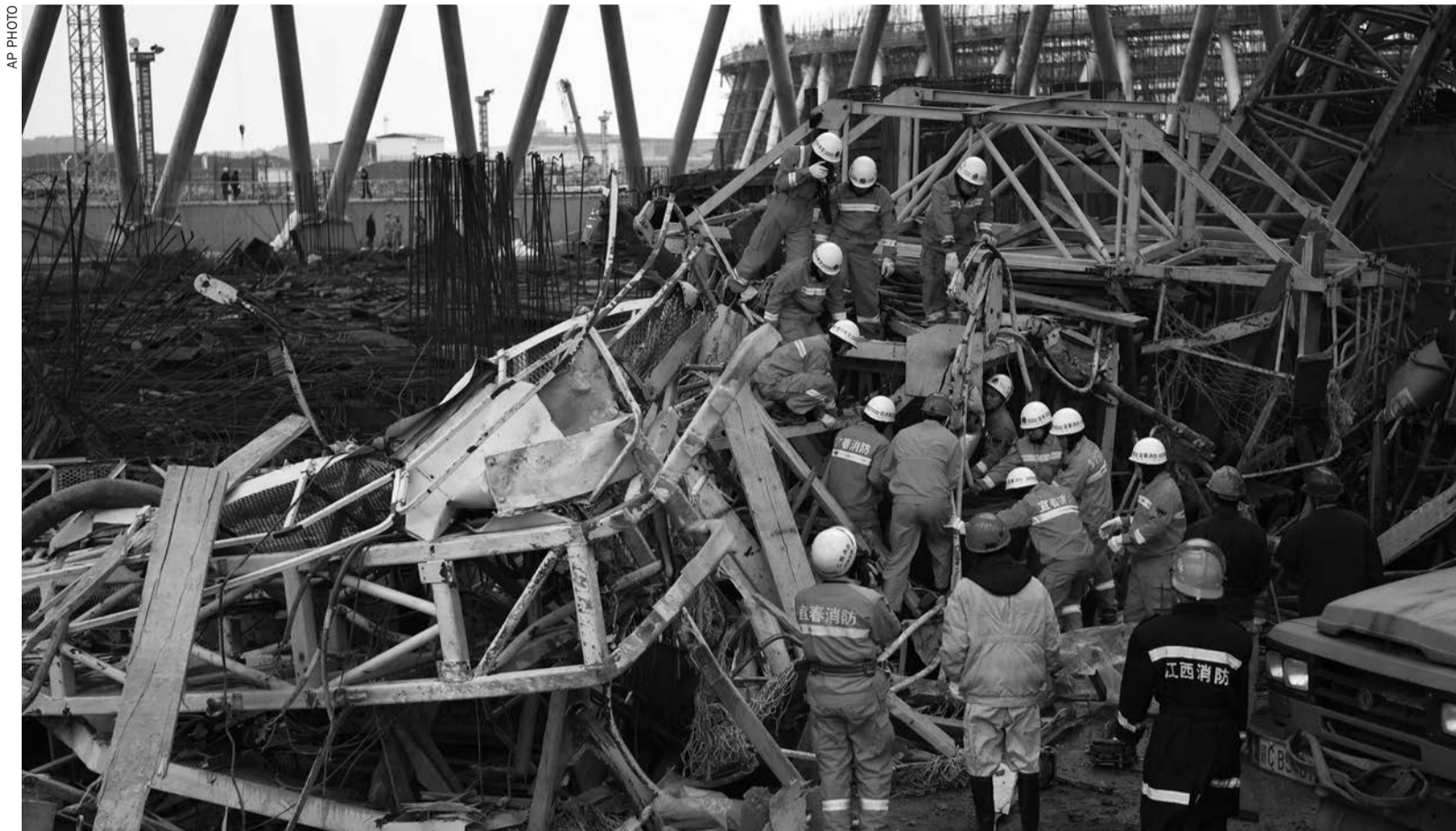
Rescue workers look for survivors after a work platform collapsed at the Fengcheng power plant in eastern China's Jiangxi Province
