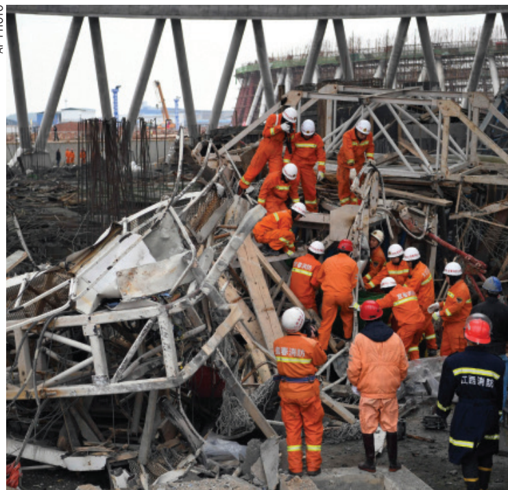
Workers look for survivors after a work platform collapsed at the Fengcheng power plant in eastern China's Jiangxi Province
