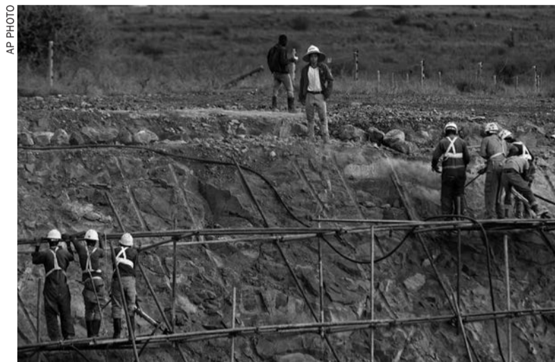
Chinese foreman supervises Kenyan laborers as they finish the sides of a cut of the Nairobi-Mombasa railway
