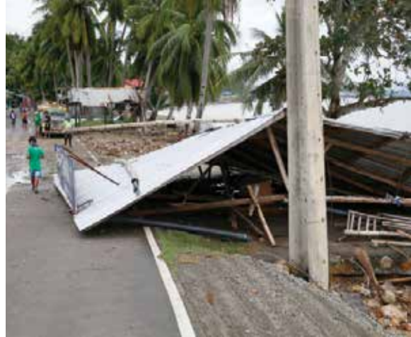
The entire roof of a store partially blocks the road after being swept by typhoon Nock-Ten
