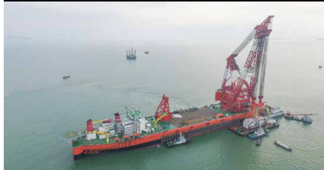
A gigantic crane, which was transformed from a tanker, hoists a 6,000-ton key structure of the world's longest cross-sea bridge linking Hong Kong, Zhuhai and Macao. The wedge, 12-meter-long and weighing more than 25 Airbus A380 jets, was lowered yesterday to connect the immersed tubes of the underground tunnel of the bridge. The 55-kilometer infrastructure includes a 22.9-km bridge and 6.7-km underground tunnel.
