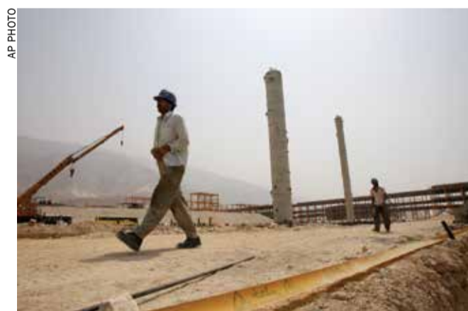
Iranian workers walk in a construction site which is part of South Pars gas field, on the northern coast of Persian Gulf
