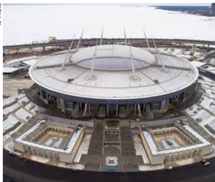
A view of the stadium under construction on Krestovsky Island, St. Petersburg
