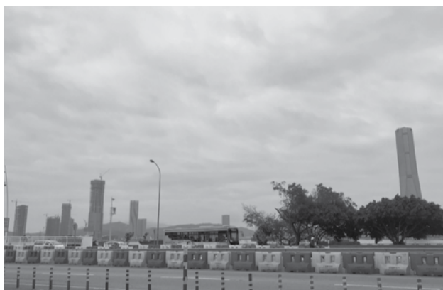
Numerous buildings are under construction close to Sai Van on the Zhuhai side of the border. Some of them emit light even before their conclusion
