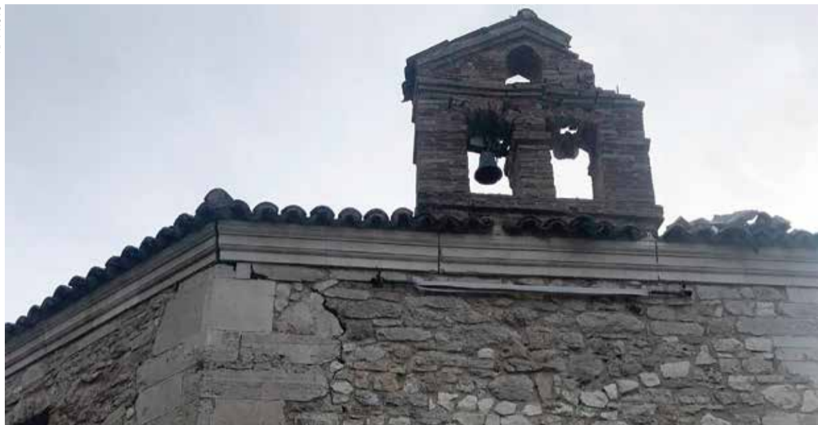
A view of a damaged bell tower of the 17th century Santa Maria di Varano' church after an earthquake, in Muccia, central Italy
