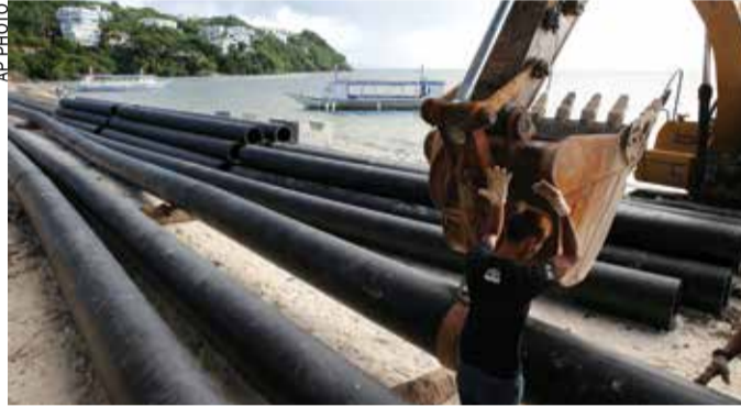
A worker signals a backhoe operator during a pipeline project along the beachfront
