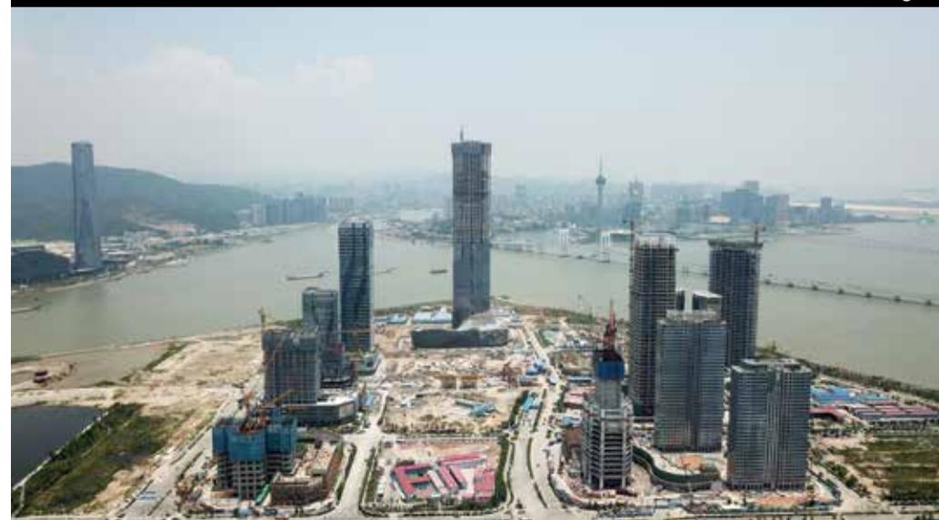
The Zhuhai Hengqin International Financial Center under construction, with Macau in the background. The main structure of the 333-meter-high building, with construction area of 218,000 square meters, was finished last month.
